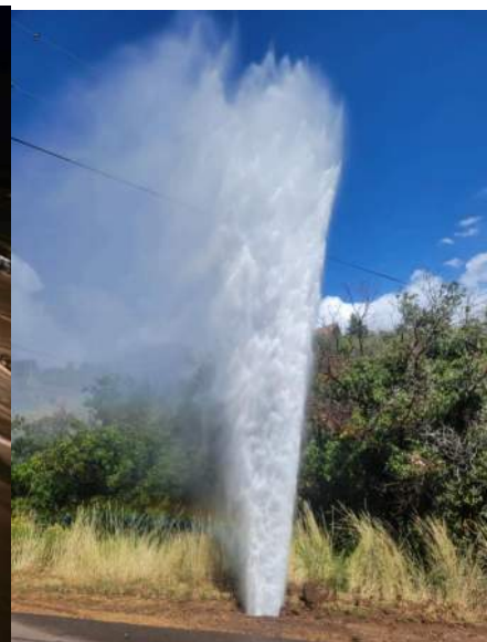
St. Moritz Water line break – 9/15/24
