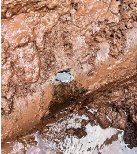
Corroded pipe section from 9/15/24 line break - Top of pipe
