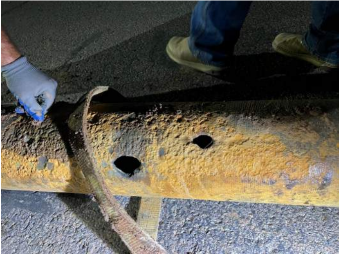
Corroded pipe section from 9/8/24 line break - Bottom of pipe
