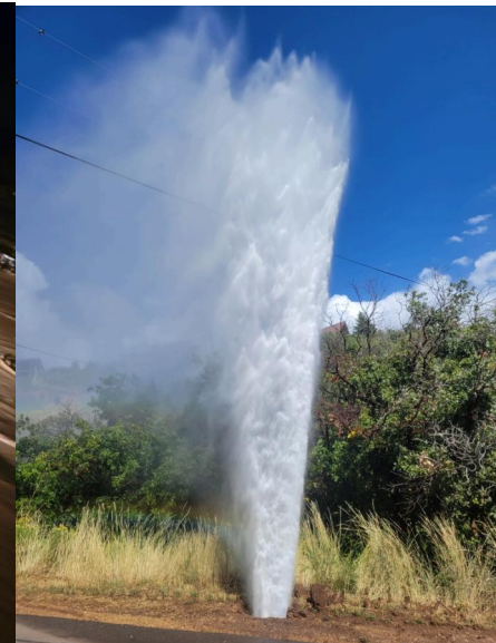
St. Moritz Water line break – 9/15/24
