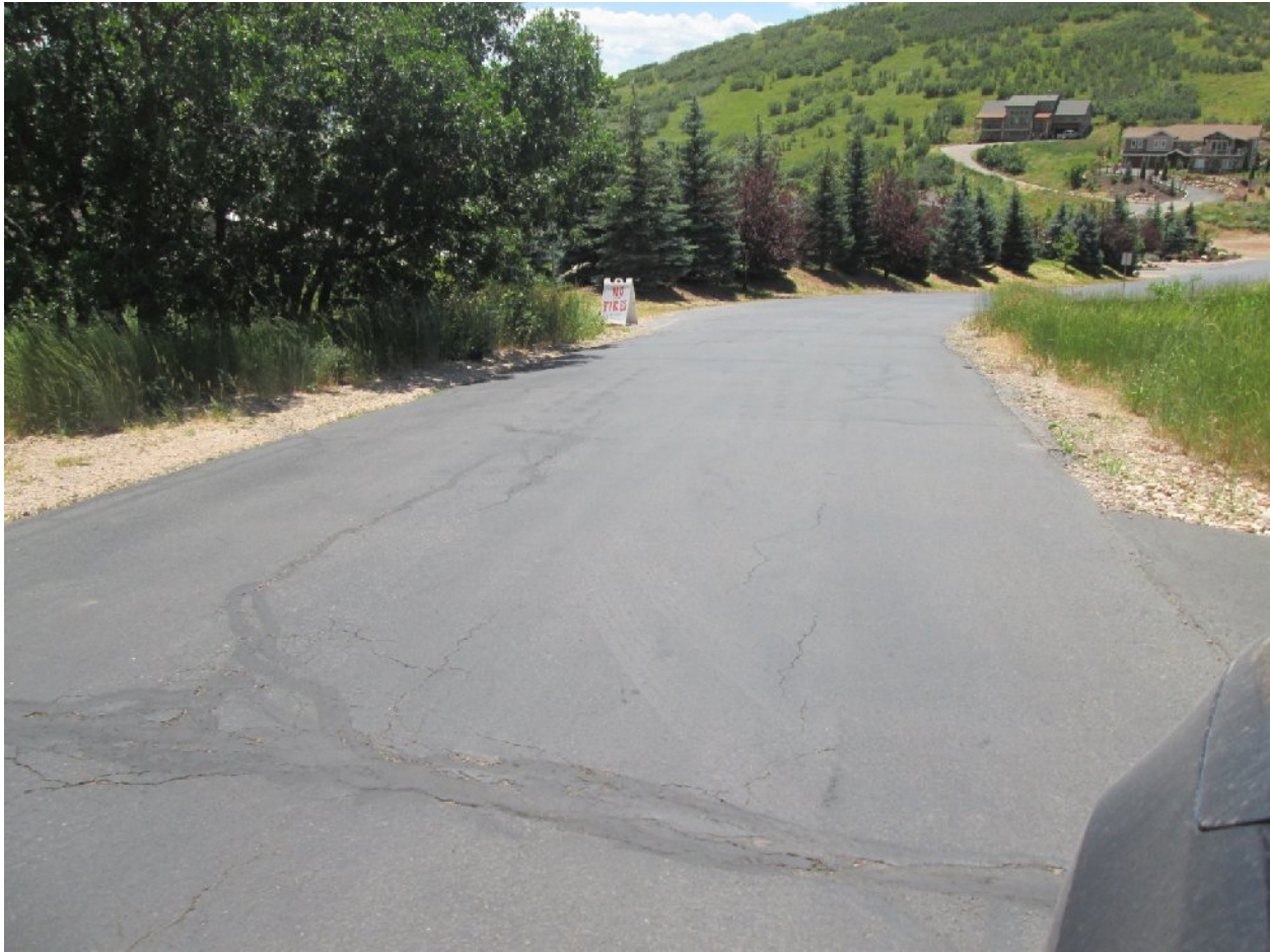
Photo 1. Fair Condition – Interlaken Dr from Interlaken Dr to Edelweiss Ln (RSL = 8 years)
