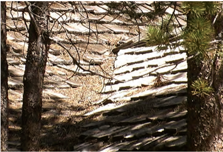
This home has a triple threat: wood shake roof, pine trees overhanging the house, and dead needles and other debris collected on the roof.
